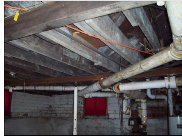
Mag Straight Run and Mag Fittings Basement
