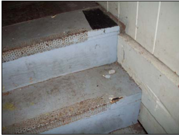
Floor Tiles w/ Mastic Basement Stairs
