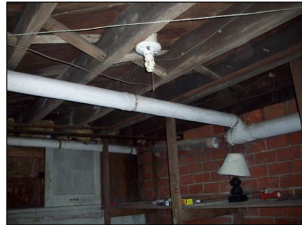
Mag Straight Run and Mag Fittings Basement
