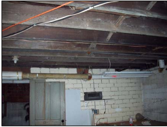
Fluorescent Lights Basement
