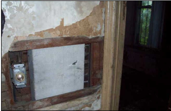
Example of Duct Wrap Straight Run from first to second floor. Dining Room/Kitchen (West Side of House)
