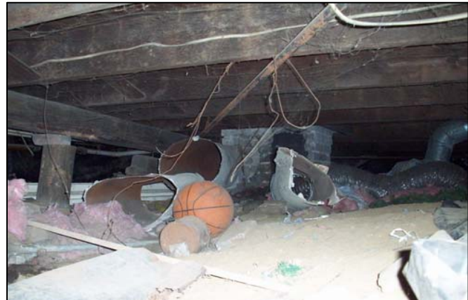
Example of Duct Wrap 16" and 10" pipes Basement/Crawl Space
