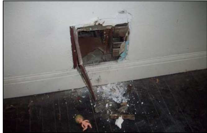
Example of Duct Wrap around Register Boot Second Floor Bedroom
