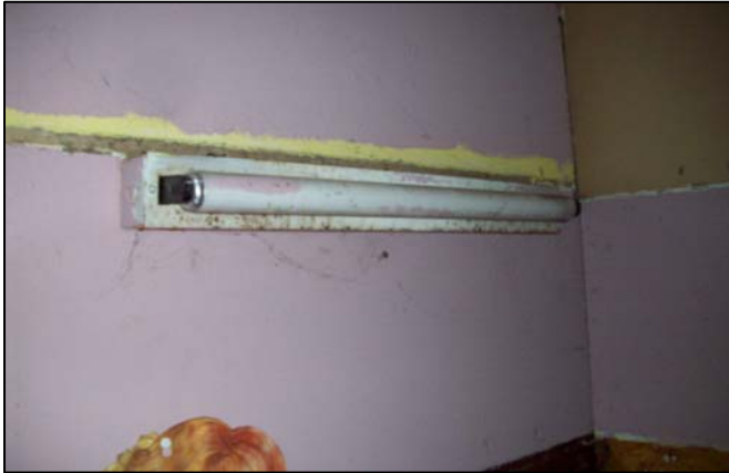
Fluorescent Light Bulbs and Ballasts Kitchen
