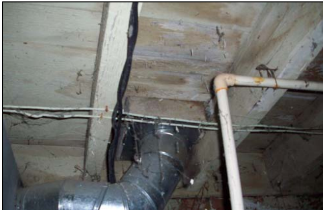
Example of Duct Wrap on Register Boot Basement/First Floor
