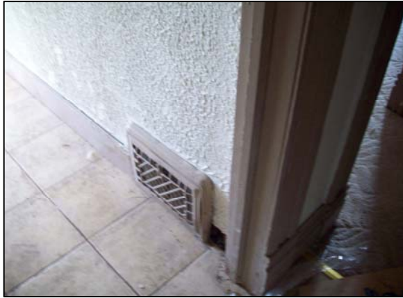
Example of Duct Wrap Register Boots/Runs Throughout
