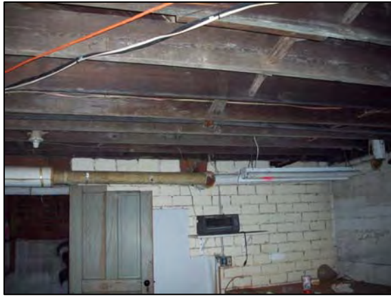
Fluorescent Lights Basement
