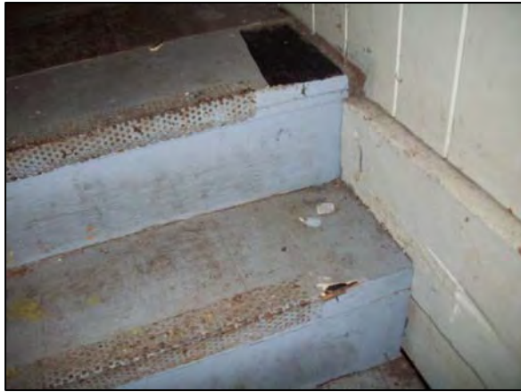
Floor Tiles w/ Mastic Basement Stairs
