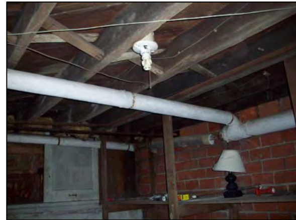
Mag Straight Run and Mag Fittings Basement
