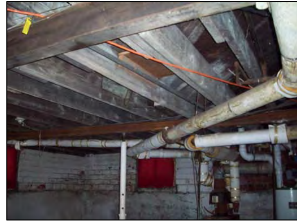
Mag Straight Run and Mag Fittings Basement
