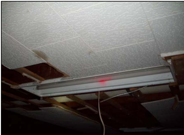
Fluorescent Lights and Ballasts Basement
