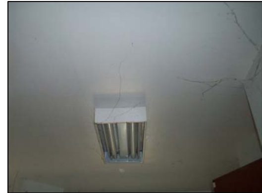
Fluorescent Lights Kitchen
