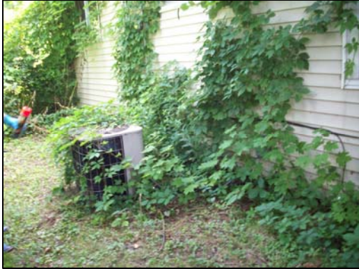
Air Conditioner Side of House
