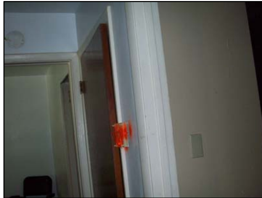
Mercury Thermostat Hallway
