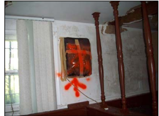
Air Conditioner Basement
