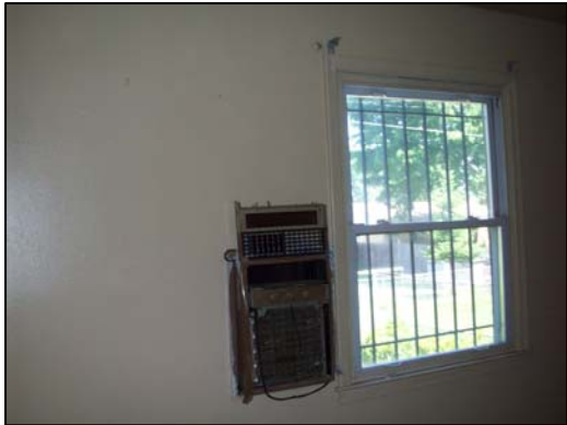
Air Conditioner Living Room
